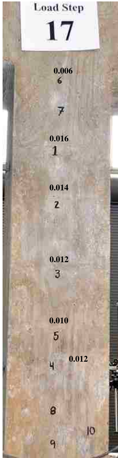
Figure 4-83: Cracks on east face of TS01 at Load Step 17
